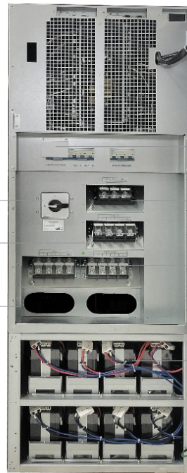
E91-40K front view (door & panels removed)
